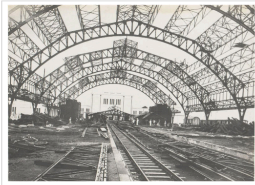
Figure 6. Station roof S.S. at Tandjong Priok under construction/span 40 meters - length 200 meters ( https://www.rijksmuseum.nl/en/collection )
