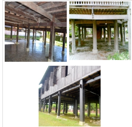
Figure 2. Composition of the lower structure of a traditional Bugis aristocratic house in Bone
