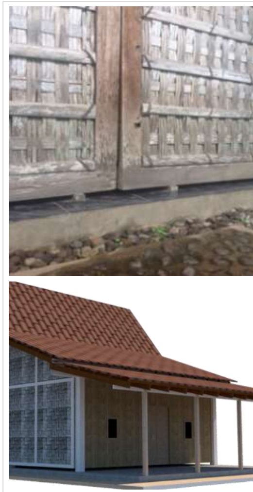
Figure 10. Construction of walls not attached to the floor in the Osing house
