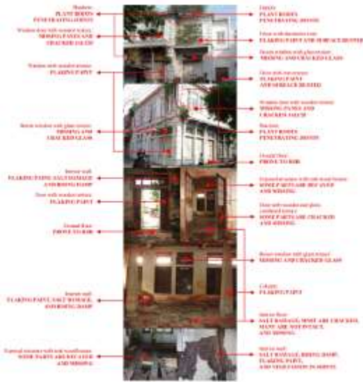
Figure 12. Significant changes in the existing exterior and interior textures due to the various types of damage before conservation
