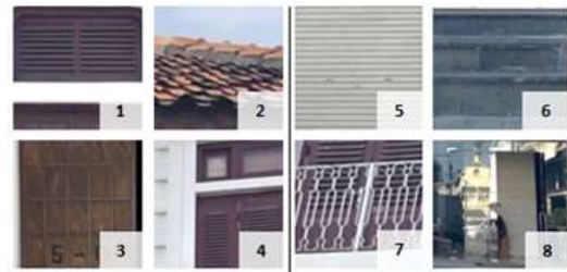
Maintained existing textures Added new textures Figure 13. The latest texture of the main facade after conservation
